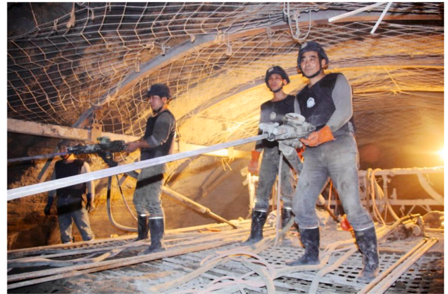
Fig. 22. Workers are equipped with bullet-proof vests and helmets to work in the strainburst-prone Micangshan Tunnel of the Bashan-Shaanxi Expressway (photo source: www.guancha.cn ).
